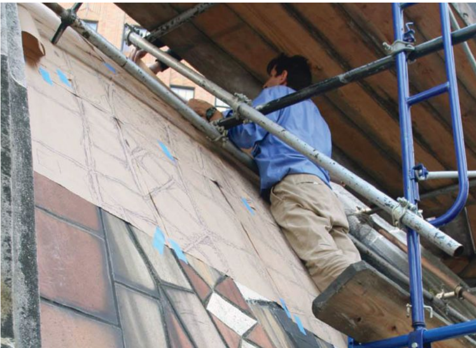
Architect Lou Martino hand traced each tile to create the dimensions and specifications for tile production.
