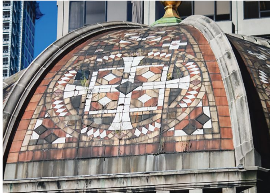
After nearly 100 years, the masonry bed of the dome had deteriorated, tiles were held in place with the aid of protective netting.
