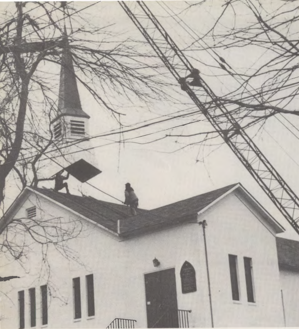
THE CROSS is fixed to the steeple of St. Simon's, New Rochelle, Dec. 21, the finishing touch to one of the new churches built under the "Cornerstone" Campaign.
